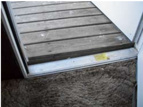
Frost caused ramp and MH to become misaligned
