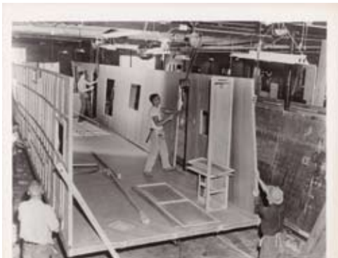
Older MHs have 1.5" walls
