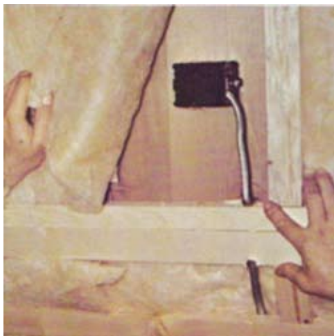
MH electrical wiring
