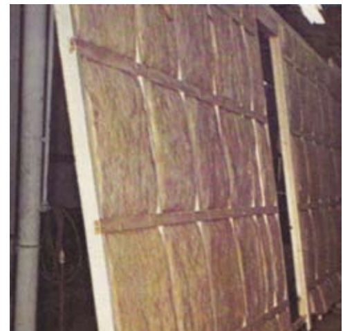
Older MHs have 2" walls
