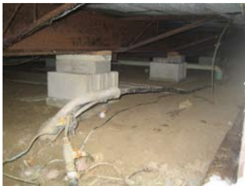
Wiring and plumbing under a Johnson County mobile home. 28 Feb. 2010.
