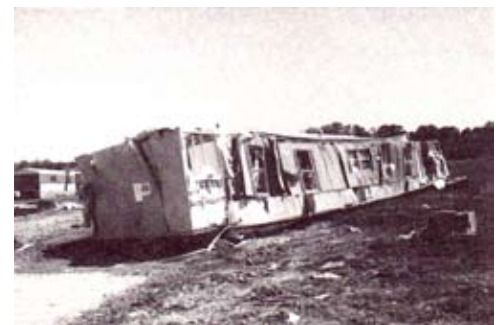
Wind damage Source: Allan Wallace
