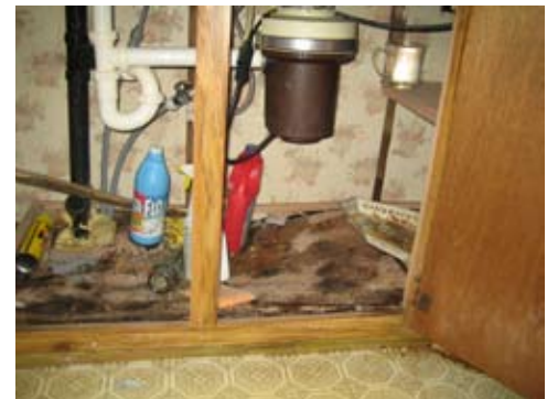
Water damage on particle board under sink
